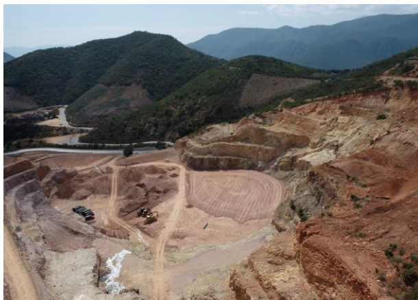
Dry Stack Tailings Filtration Plant and Dry Stack Area
